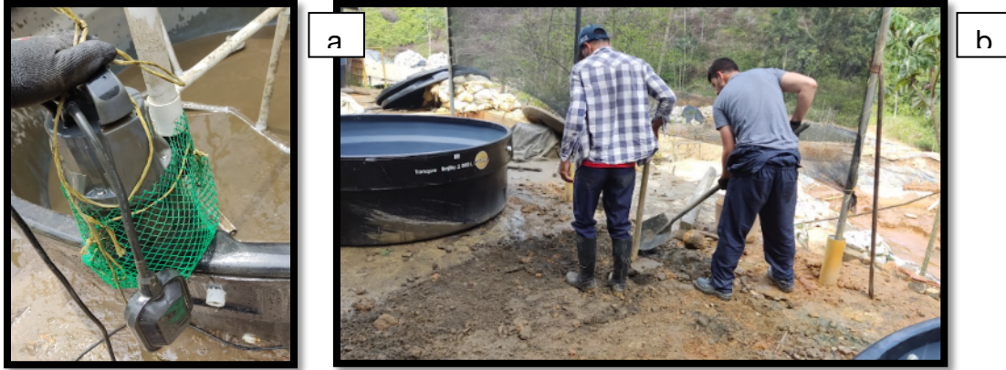
Figure 7. Adaptation of the location for assembly; a) Securing of solids pumps, b) Suitability of the land. Source: Pure Earth, 2023.
